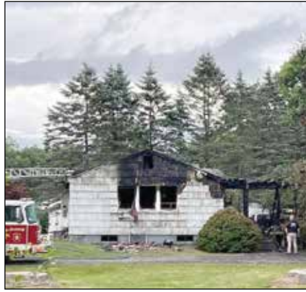
Fire damage to the house at 42 Daniel Square.
